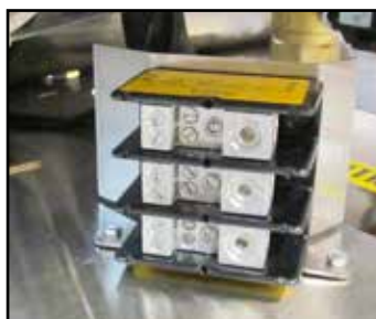
Fig. 3 - Booster terminal block
