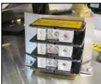
Fig. 18 - Booster terminal block
